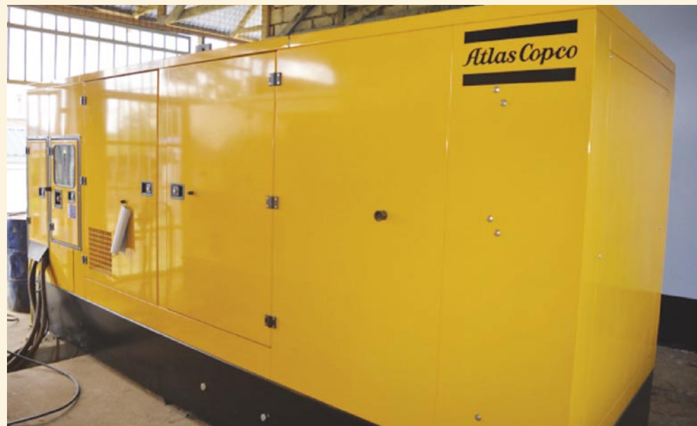
Meru Teaching and Referral Hospital backup generator.
