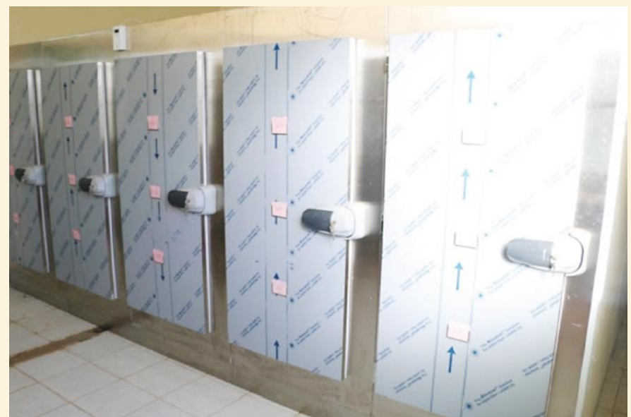
Ultra-Modern Nyambene level 4 hospital mortuary (Cold room) which has the capacity of 30 bodies.
