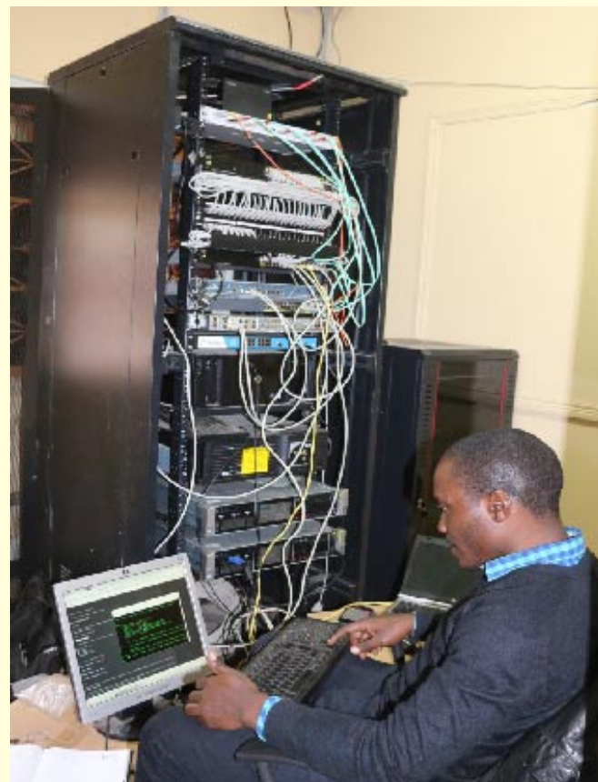
Meru County Government Server room.
